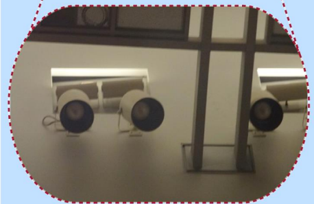
Ronald Reagan Federal Building and Courthouse (Santa Ana, CA) – Lights difficult to access and replace due to seating below and slope of floor. Requires a special equipment to replace.
