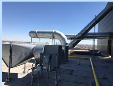
Albert Armendariz, Sr., U.S. Courthouse (El Paso, TX) – The heating, ventilation, and air conditioning chillers are located on the roof, which requires pumping water up 8 floors from the basement.
