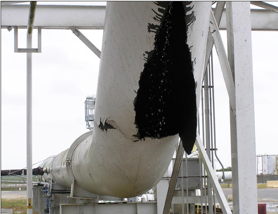
Figure 1: Strategic Petroleum Reserve, Big Hill Site – Raw Water Pipe Failure in April 2016
