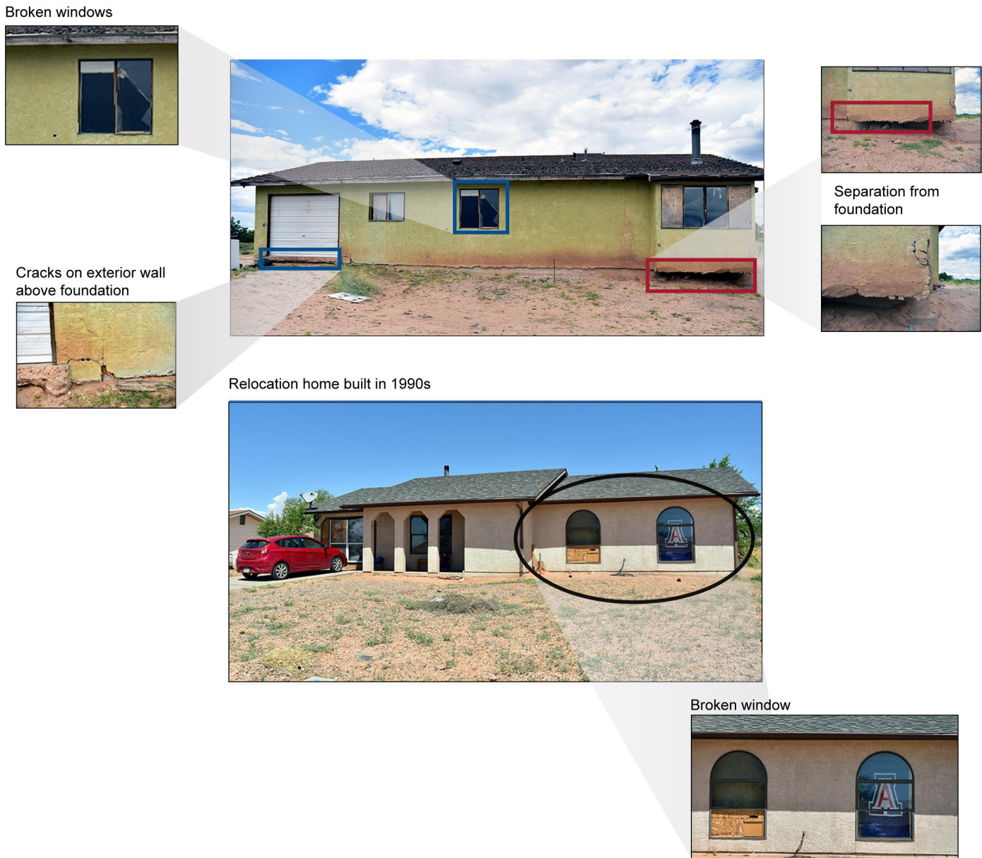
Figure 7: Examples of Homes on the Navajo Reservation with Cracked Foundations and Broken Windows
