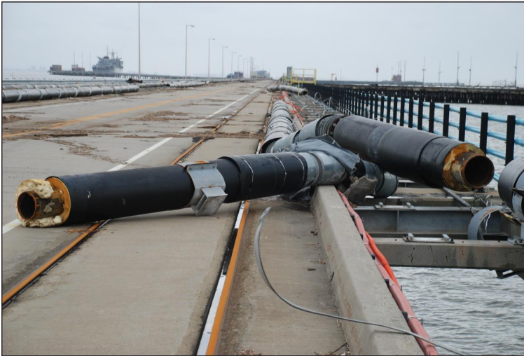
Destroyed by Hurricane Sandy
