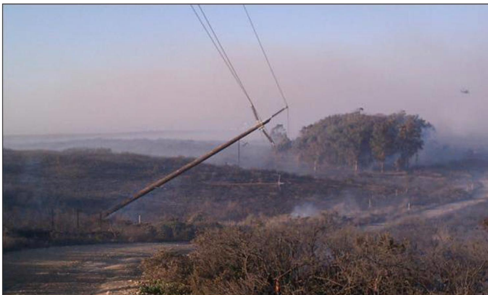
Figure 5: Utility Pole Damaged by a Wildfire on Vandenberg Air Force Base
