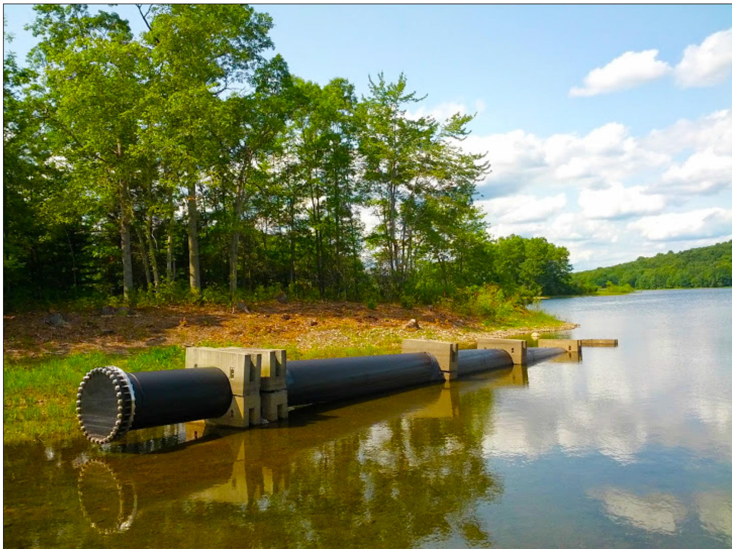
Figure 2: Improvements to Access Pipe for a Drinking Water Treatment Plant Near New London, Connecticut
