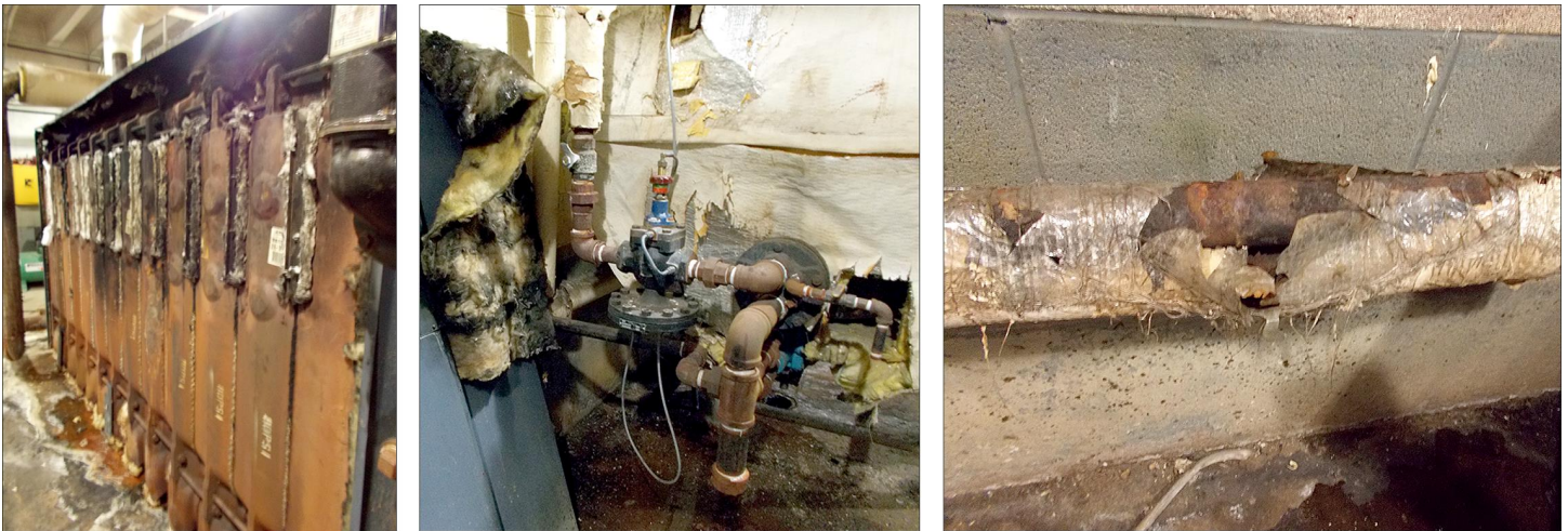
Figure 2: Aging Boiler Systems at a BIE-Operated School Built in 1959
