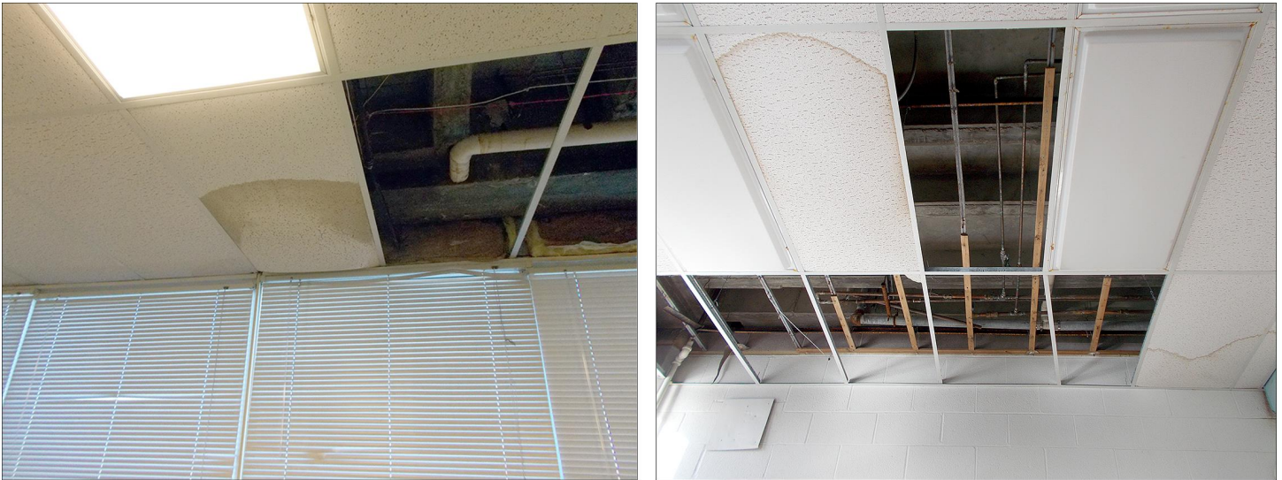
Figure 7: Damaged or Removed Classroom Ceiling Tiles Due to Leaks in Recently-Installed Roofs
