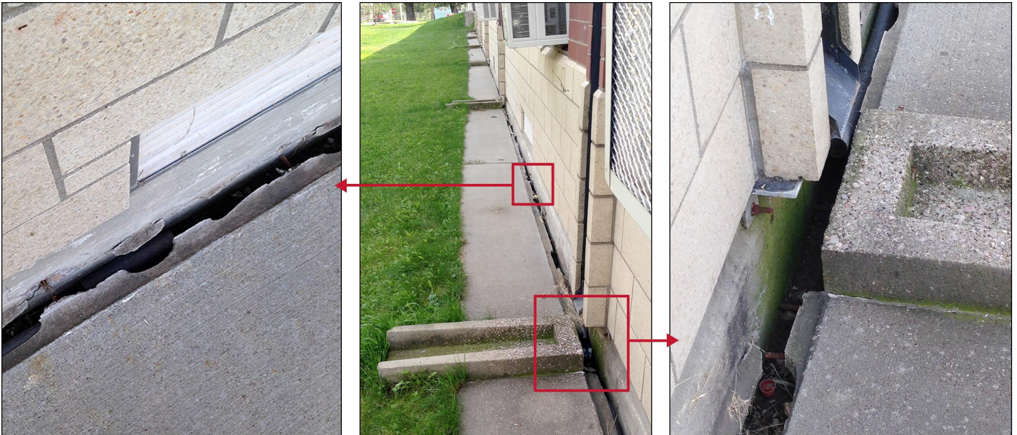
Figure 4: Building Damage Caused by Poorly Maintained Rainspouts at BIE-Operated School
