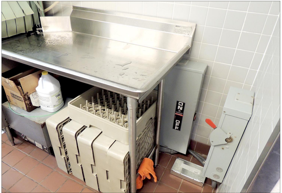
Figure 6: High Voltage Electrical Panel Installed Next to Cafeteria Dishwasher at a BIE-Operated School, October 2014
