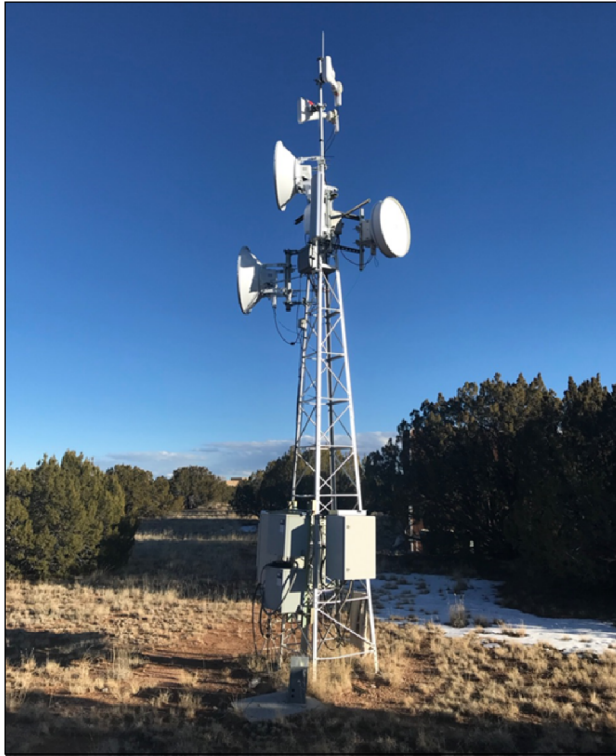
Figure 6: Example of Fixed Wireless Tower Providing Middle-mile Service in Low Population Areas of Rural New Mexico
